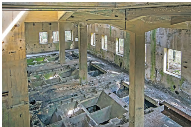
Inside one of the two main production buildings (E1 & E2) at the Dynamit factory. We couldn't work out the processes or work flow routes; research on the internet gives very little about the area
